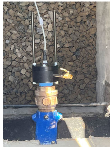
Figure 3. Sensor installed at the Gainesville pilot site on a corporation stop valve.
