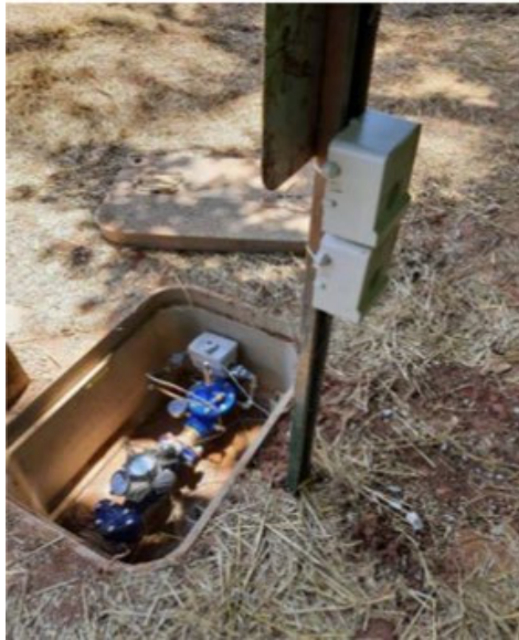
Figure 1. Gainesville's remote flush valve installation with Sensus ally meter for remote control and volume tracking.
